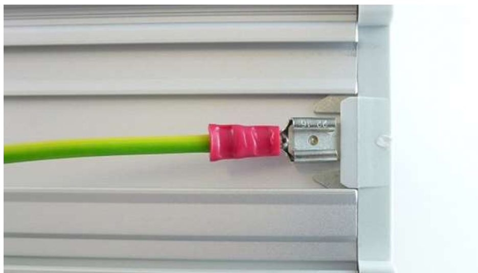
Figure 16: DIN rail housing with grounding connection (PE)
